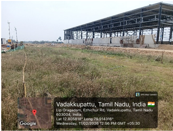
IOCL LINE AREA- SAFETY LINE
