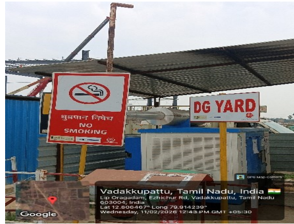
DG WITH STACK LOCATION
