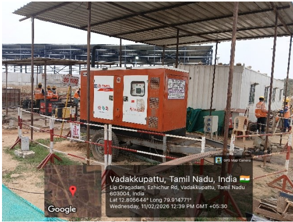
DG WITH STACK LOCATION
