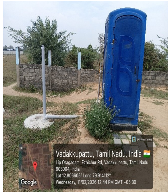
RESTROOM WITH SOAKPIT
