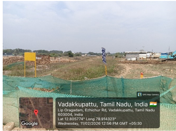
IOCL LINE AREA- SAFETY LINE
