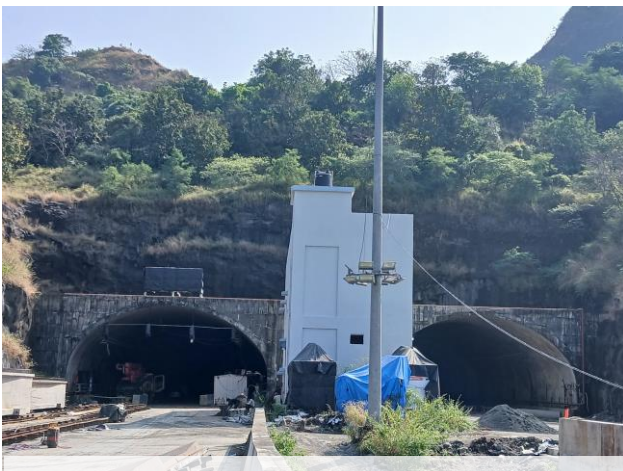
Tunnel which is in Part B is largely complete, work underway on exit side
